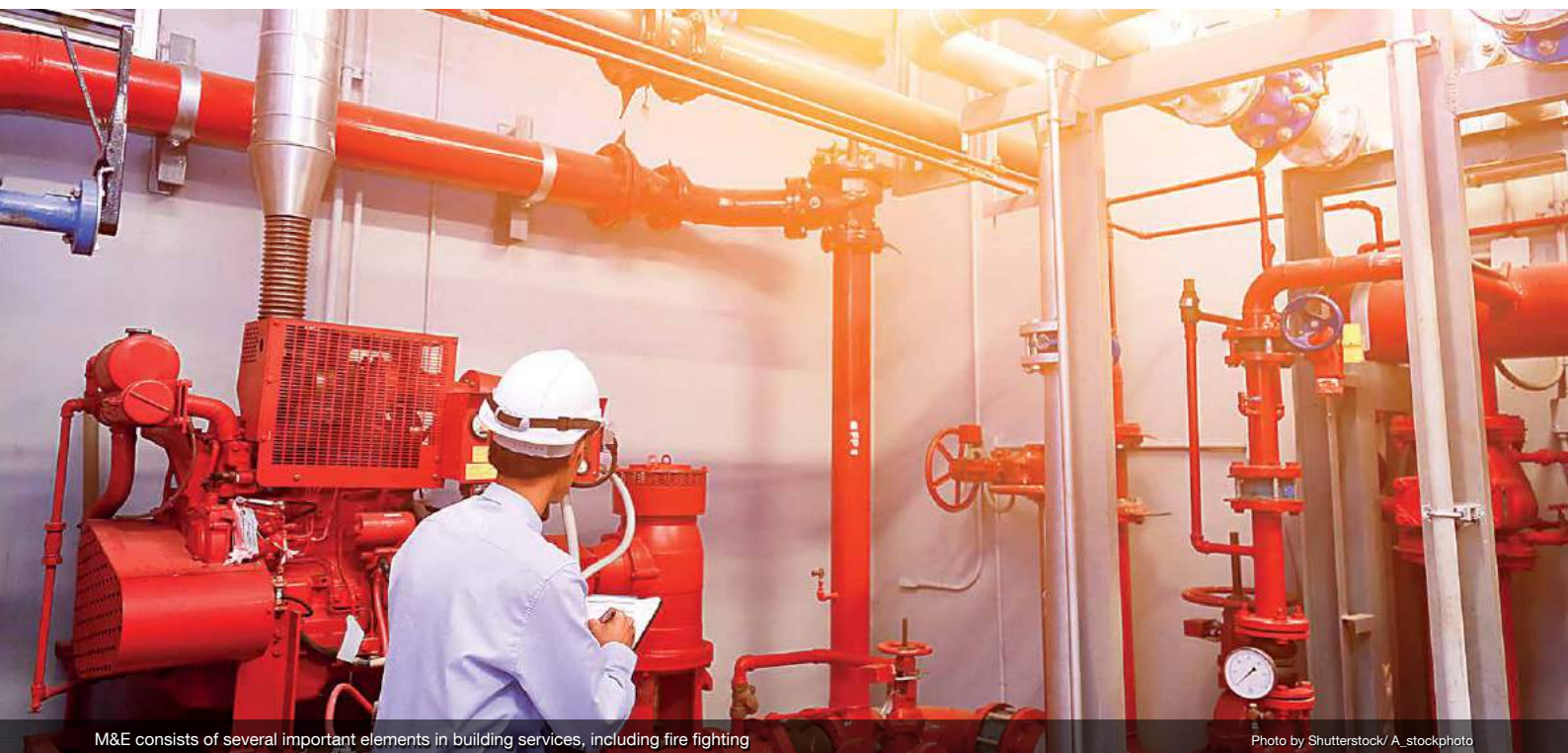
M&E consists of several important elements in building services, including fire fighting
