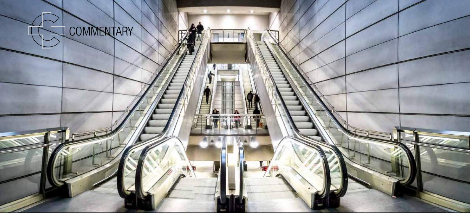
Mechanical services consist of vertical transportation, including escalator systems
