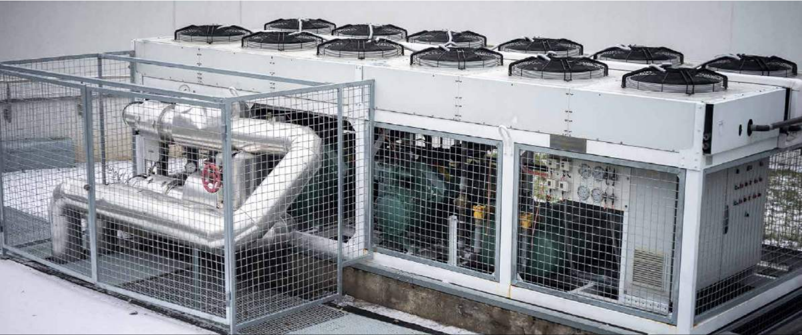
Air-conditioning technology with variable refrigerant volume/flow (VRV/VRF) will also help the architects in the design process
